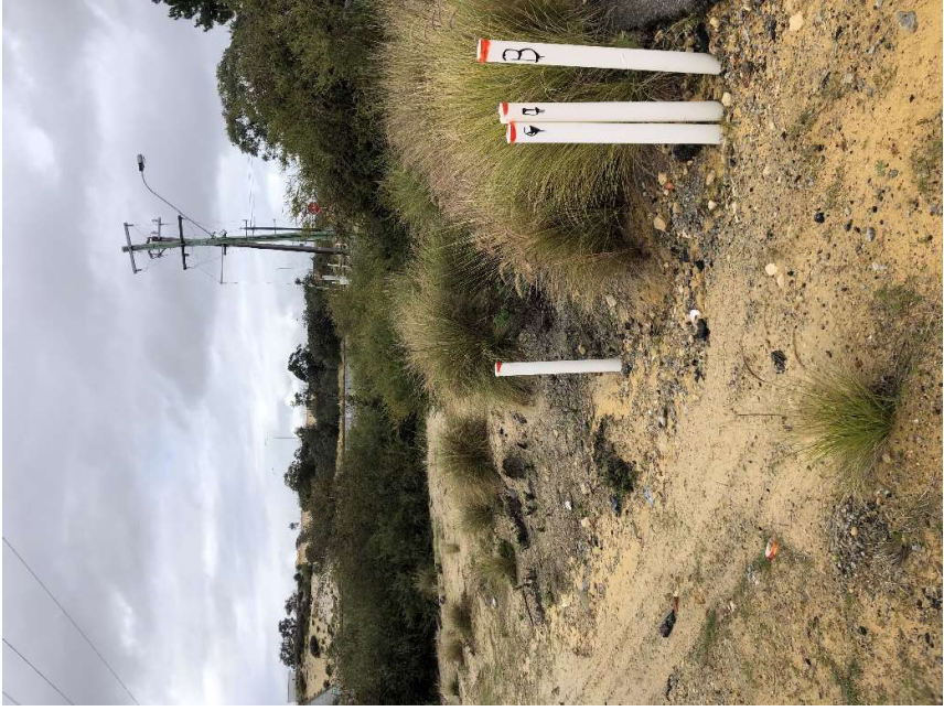
Photograph 20-1: Cleared access track on the road verge northeast of Hope Road. Vegetation consisted predominantly of exotic Cenchrus grasses with some isolated Acacia shrubs.
